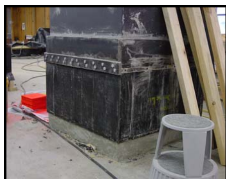
Lead rubber bearing in place at base of column
