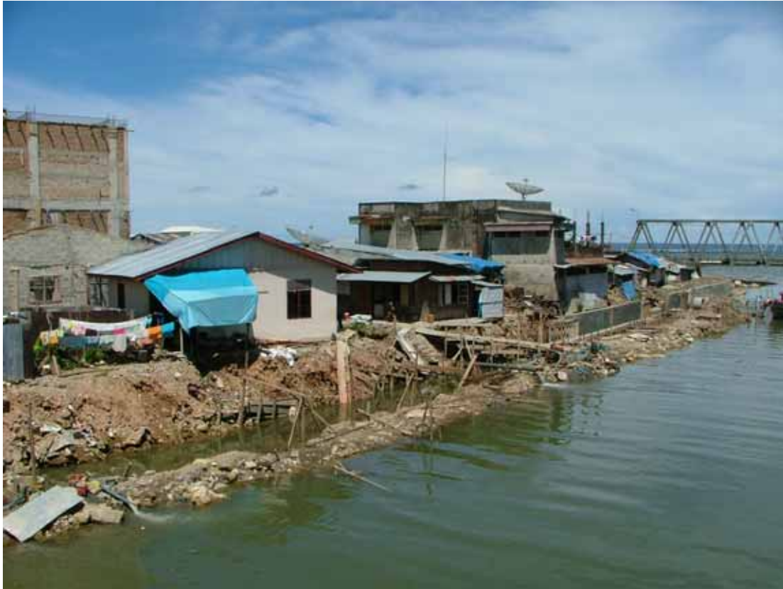
By December 2006 the buildings are nearly finished and a reinforced concrete river bank wall is being constructed. As well as the new building construction, all the roads in this area have been rebuilt.
