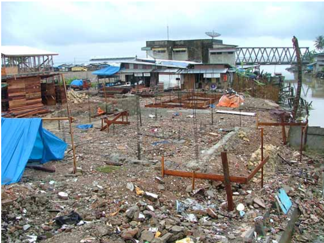
Just one of the original buildings in this part of central Gunung Sitoli survived the great earthquake shaking, but new buildings are starting to grow from the earthquake rubble in February 2006.
